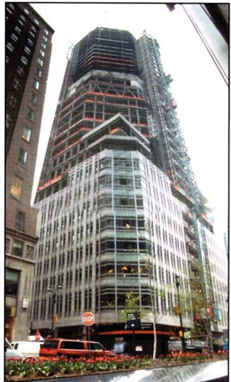
One of the many large-scale projects awarded to ADF in New York City, the 45-storey office tower at 383 Madison Avenue, required 18,000 tons of heavy built-up structural steel and was completed within 16 months.
