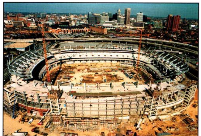
Baltimore Ravens' NFL Football Stadium in Maryland. One of ADF fast-track project, this 68,900-seat stadium required 8,500 tons of structural steel.
